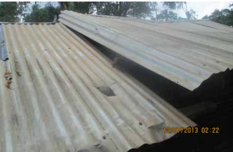
Fig (5.3): Roof of one of the affected houses.
