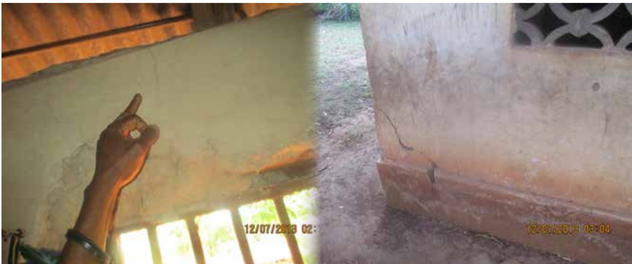
Fig (5.2): Cracks on walls of two buildings near Chauringo quarry.
